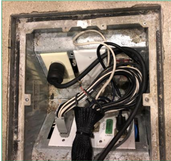
Acceptable: Floor box with all cables terminated at connection plates.
