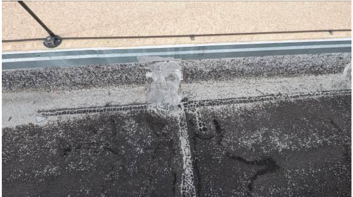
Silver coat on parapet walls that came back with a Trace that was successfully point counted below 1%
