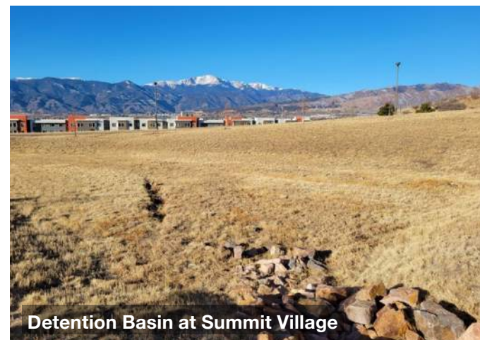
Stone Weirs in Arroyo at Summit Village
